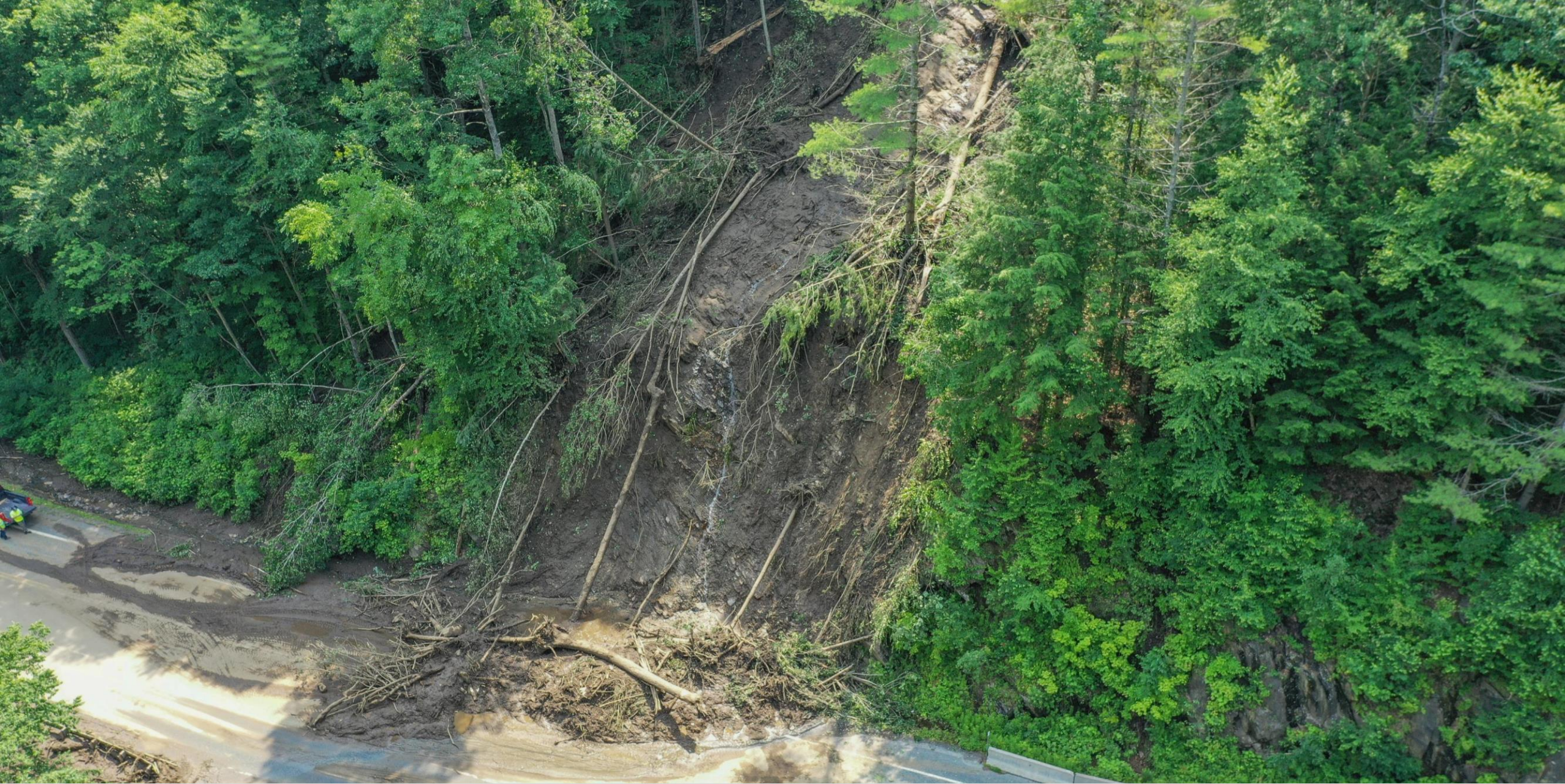
Reading VT106 Washout
