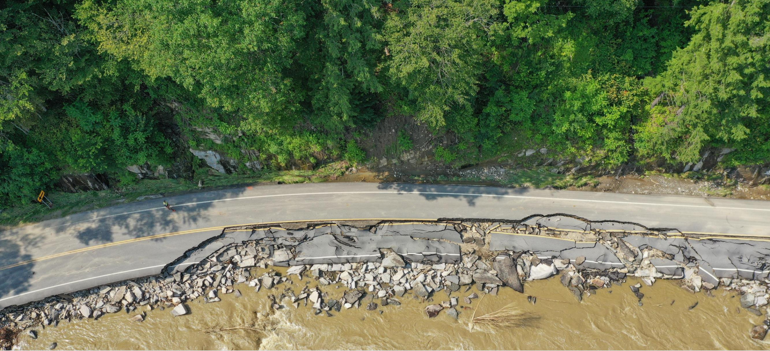
Cavendish VT106 Washout
