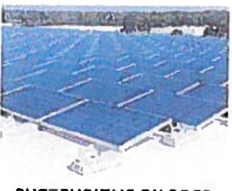
PHOTOVOLTAIC ON ROOF
